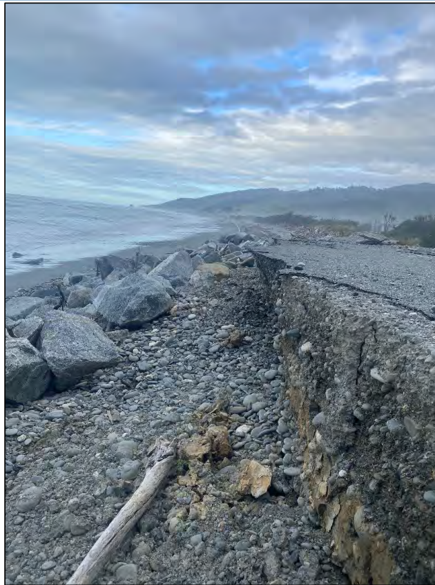
Figure 2-4 - Severe erosion of wall, with rock protection falling away from the wall completely
