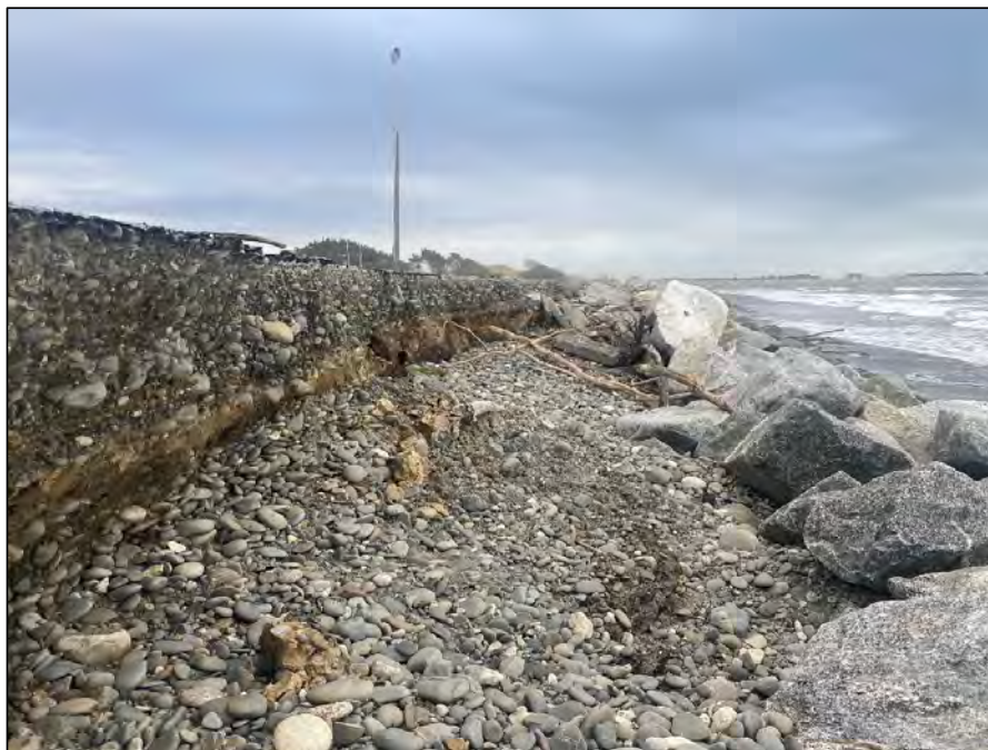
Figure 2-3 – Severe erosion of the wall
