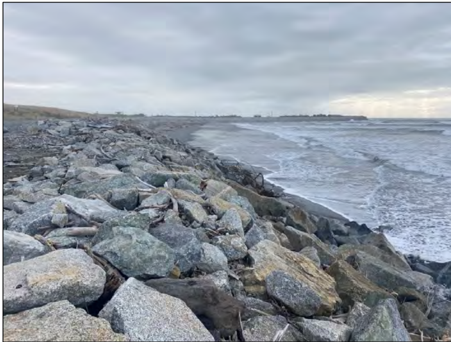
Figure 2-1 – Southern most section of wall in good condition (close to Cobden cut)
