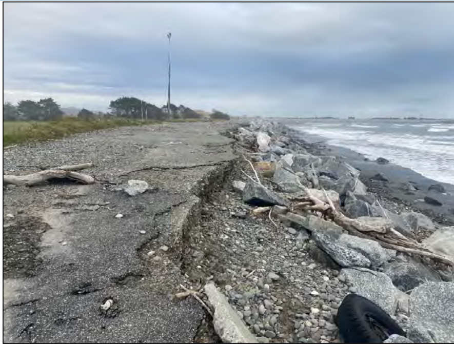
Figure 2-2 – Mid section of wall, collapsing and in serious need of repair (adjacent to Jellyman park)
