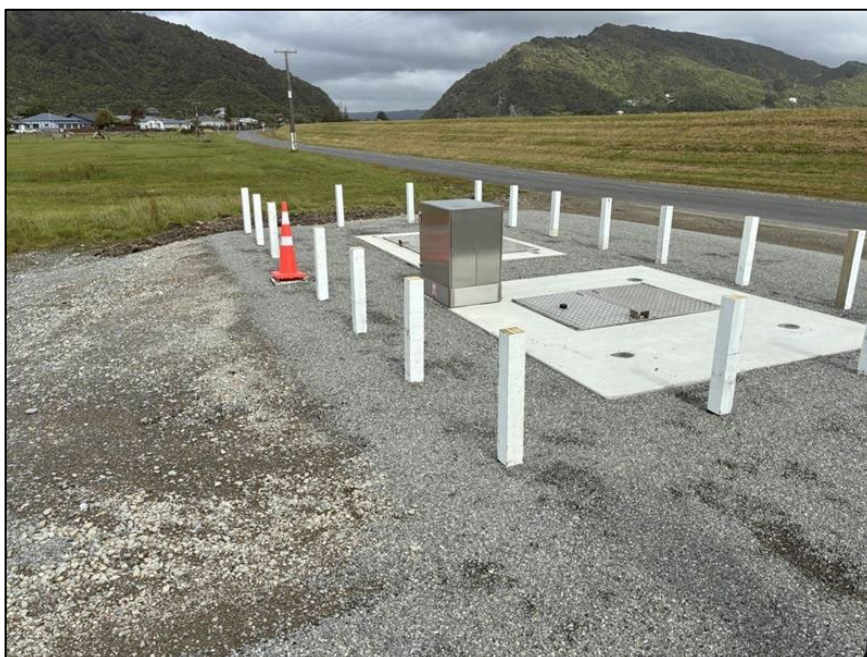
Fig 7: Cobden Wastewater Pump Station
