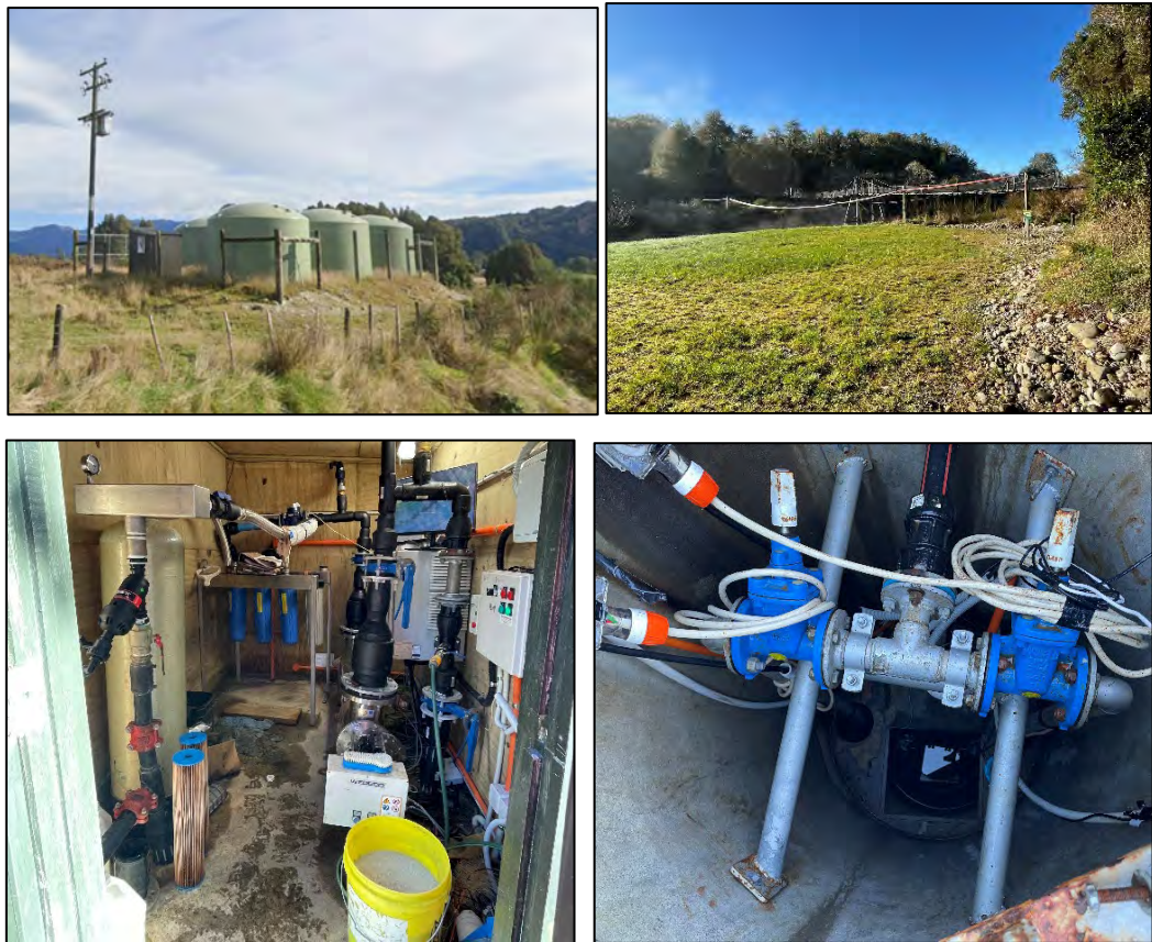
Fig 8: Selection of photos from the Nelson Creek Water Supply.
