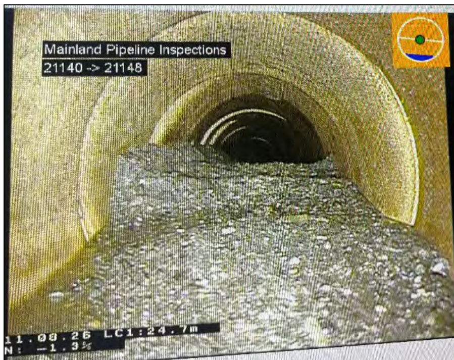
Fig 10 Debris in Stormwater network – Guinness Street
