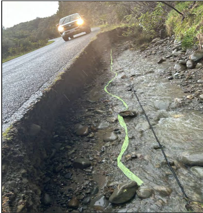
Fig 5: Erosion – McLean’s Pit Road
