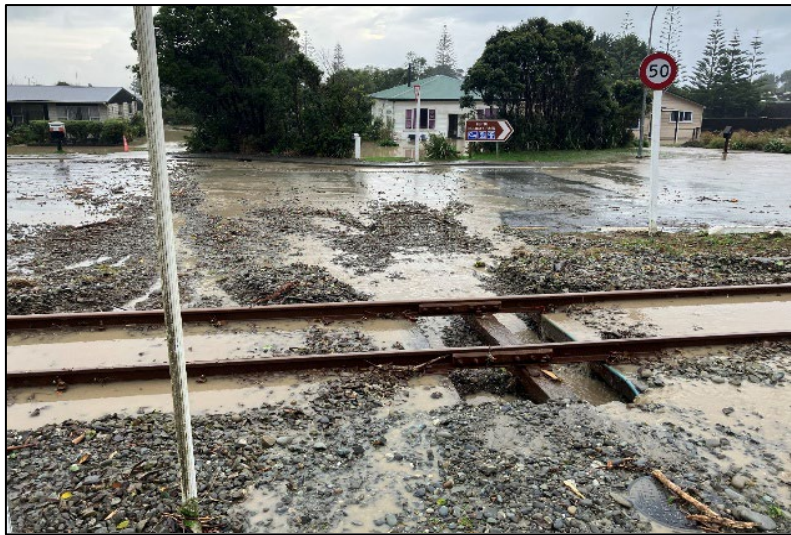
Fig 8a: Rail damage adjacent to the Tasman street/SH6 intersection, Karoro
