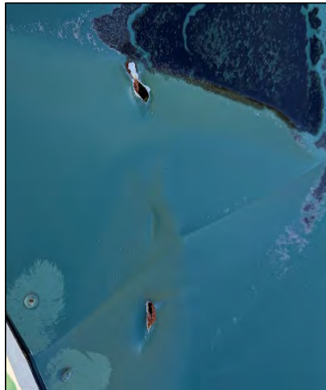
Fig 6: Bullet hole in reservoir roof
