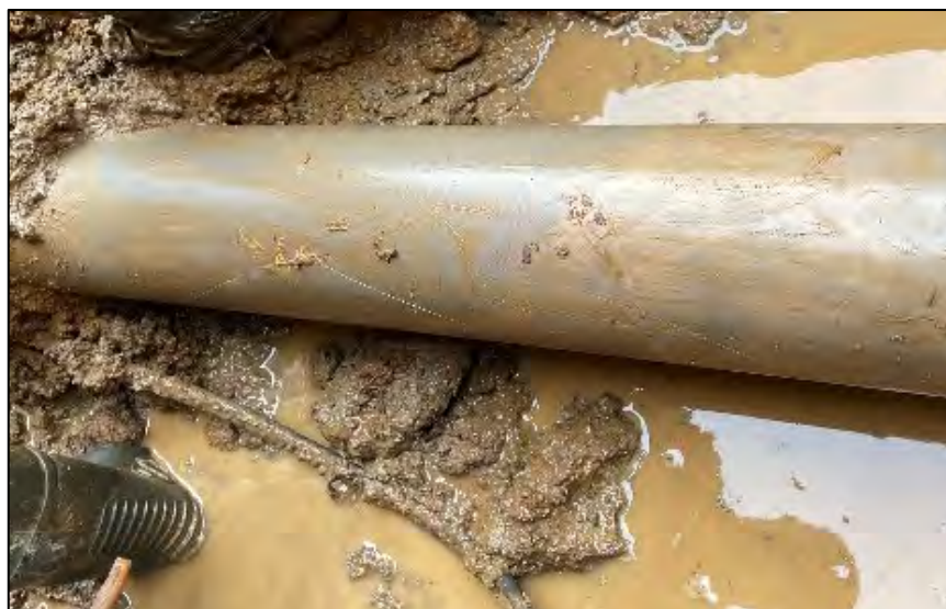
Fig 7: Damage to main during cable theft
