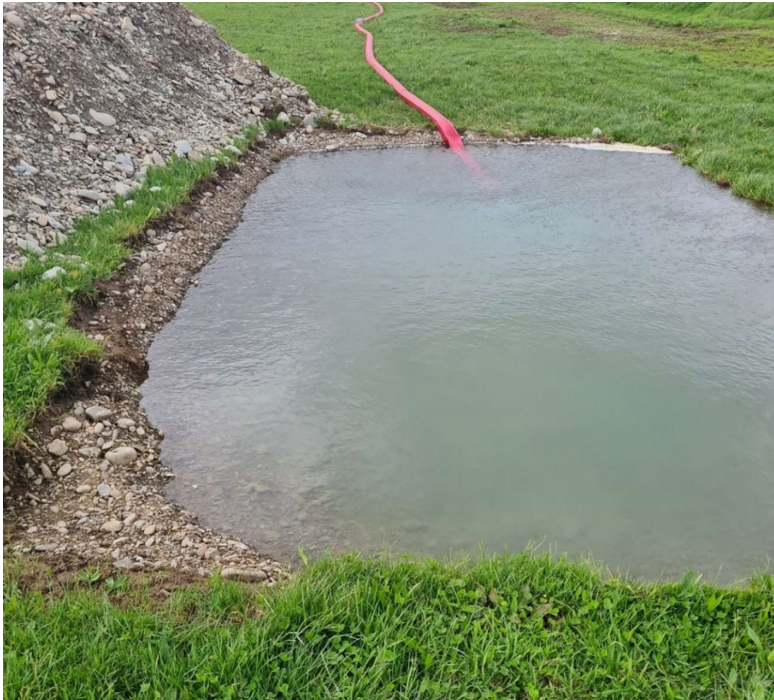
Figure 31: Infiltration trench following filling to the brim and holding at a pump rate of 25 L/s (10:40 am)
