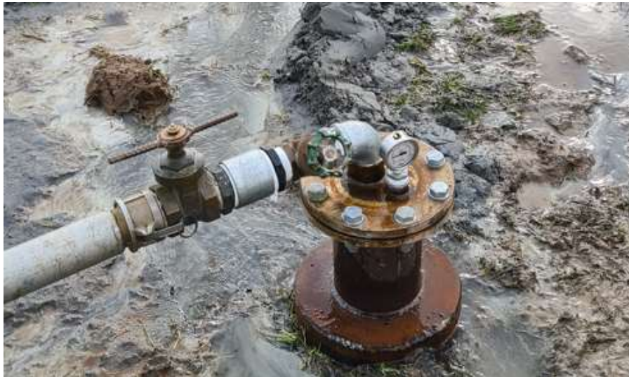
Figure 16: Headworks connected to injection circuit, including surface pressure gauge
