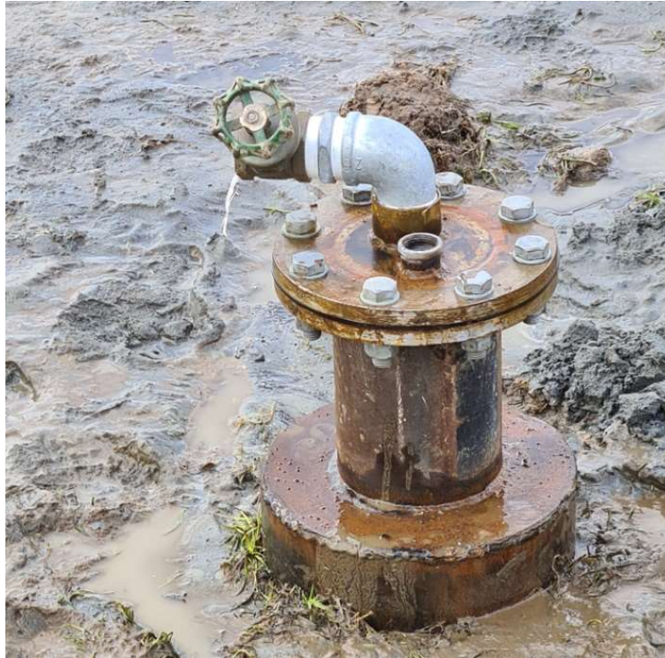
Figure 15: Injection well headworks, including welded outer & inner casing and flanged cap
