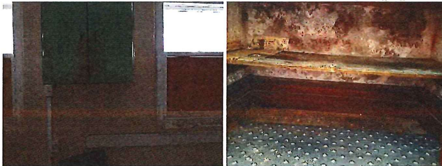
Figure 11. Dampness of Internal Walls
