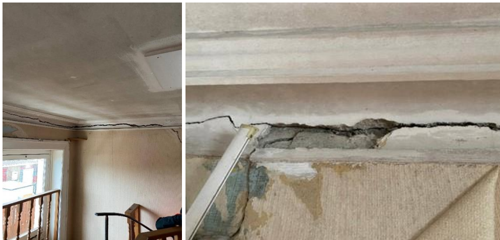
Figure 4. Cracking along top interior edge of perimeter walls
