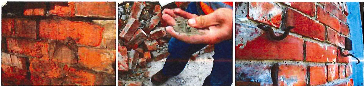
Figure 18. Deterioration of URM Wall Elements (NZSEE Guidelines)
