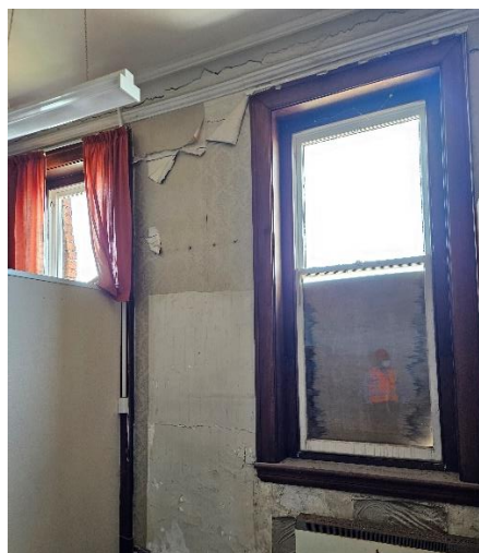
Horizontal crack above window head
