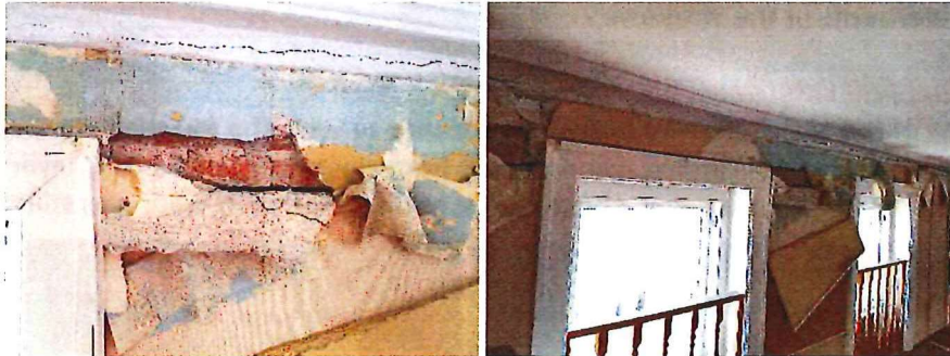
Figure 10. Cracking of the Internal Perimeter Walls
