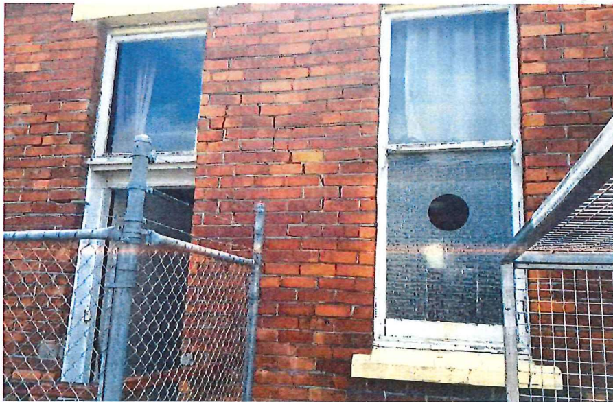
Figure 26. Cracking in Brick Veneer
