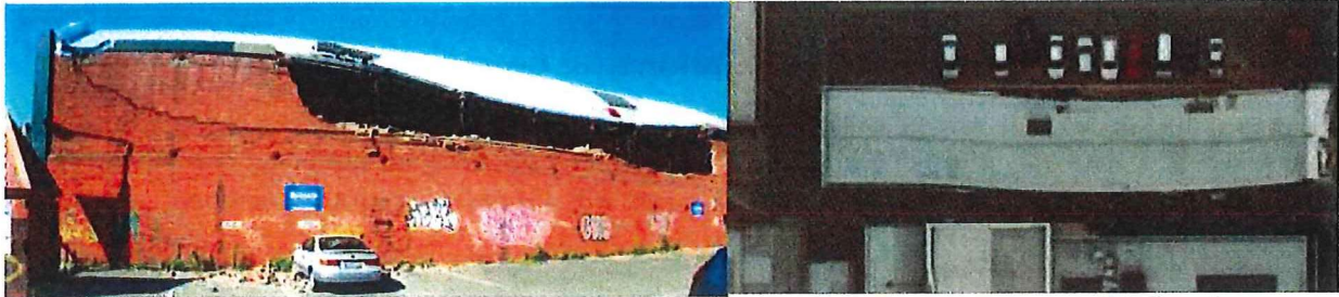
Figure 15. OOP Failure due to Diaphragm Displacement (NZSEE Guidelines)
