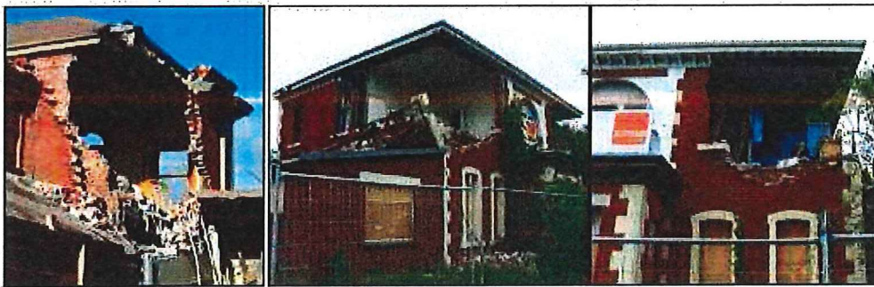
Figure 16. Examples of Building Corner Failures (BRANZ)
