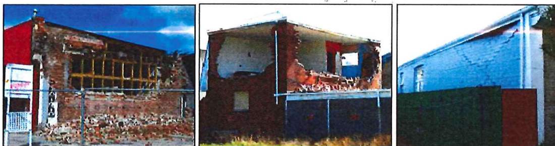
Figure 13. OOP Failure of URM Wall (BRANZ)
