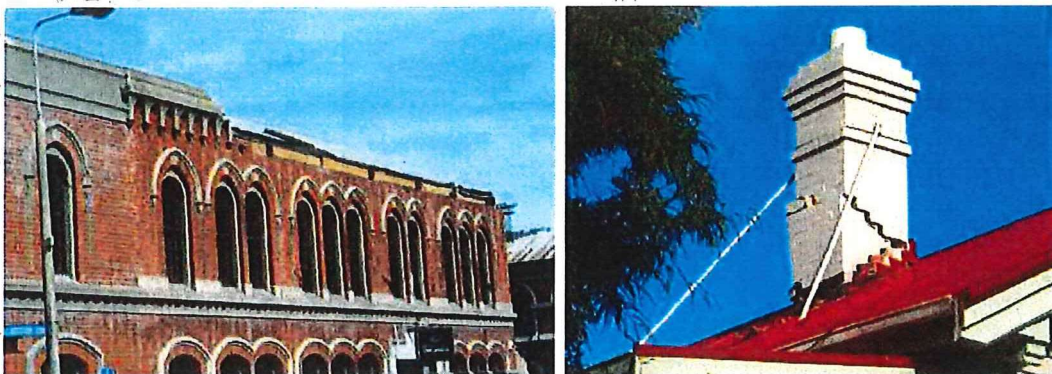
Figure 17. Failure of Secondary Elements (NZSEE Guidelines)
