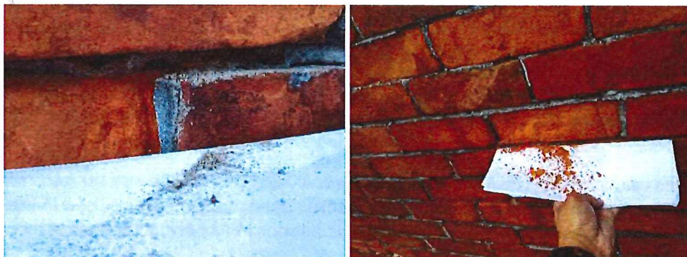
Figure 20. Condition of Bricks and Mortar on Exterior Veneer
