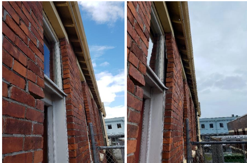
Figure 2. Visible bowing in western external façade. The 2019 photo is shown on the left for comparison
