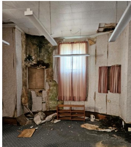
Signs of mould and water ingress
