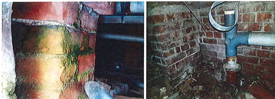
Figure 7. Damp Foundations with DPC Layer
