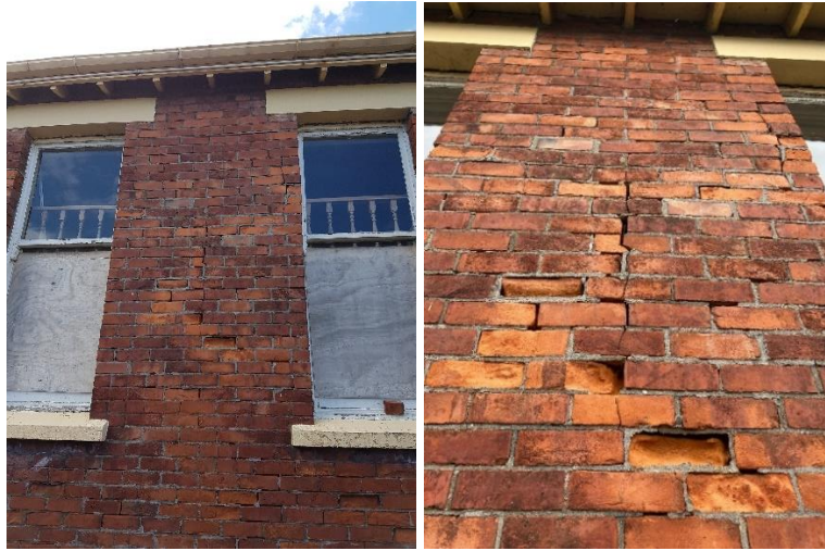
Figure 1. Significant cracks in western external façade. The 2019 photo is shown on the left for comparison
