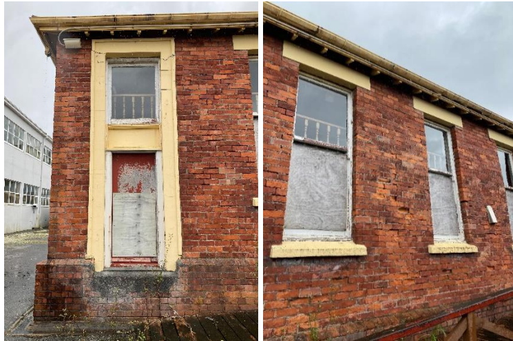
Figure 3. Cracks to external concrete lintels
