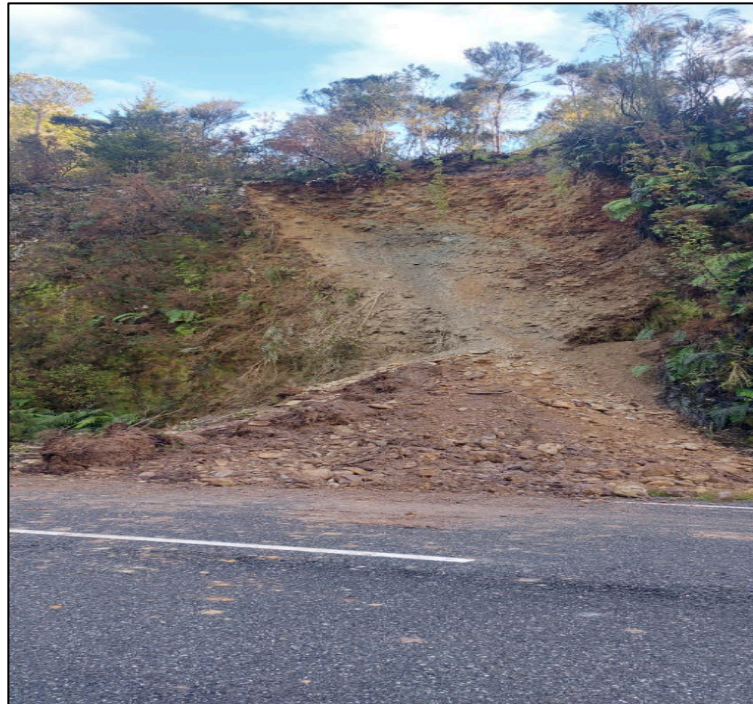
Figure 11: Minor Slip Taramakau Valley Road
