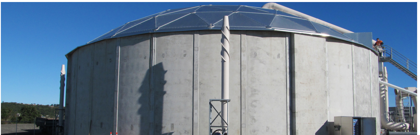
Greymouth wastewater treatment plant in Preston Road
