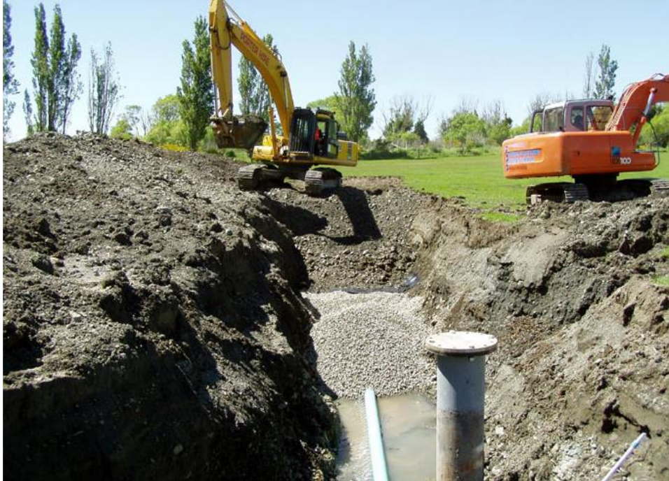
Figure 52: Example of infiltration gallery construction [photo credits to Butt Drilling Ltd (buttdrilling.co.nz)]
